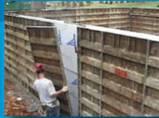
STEP 3: Place reinforcing bars in the slots provided in the ThermaEZE webs or on the notched wall ties and you're ready to pour.
