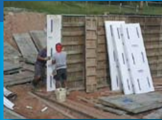
STEP 2: Install ThermaEZE panels into wall cavity as you erect your wall forms.*
